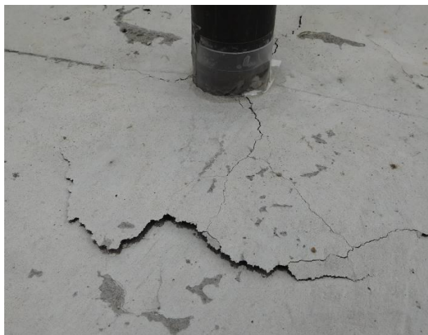
Figure 19. Early concrete surface cracking
