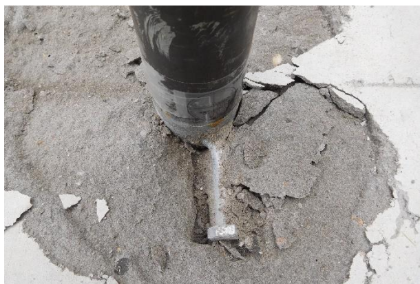
Figure 18. Concrete failure of stud connection
